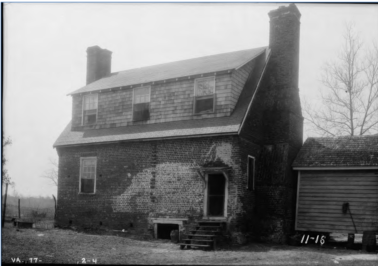
Rear elevation of Lynnhaven House, ca. 1936, showing the same brick racking illustrated by the photo above, along with surviving plaster on the rear wall. Image courtesy of HABS/Library of Congress.
