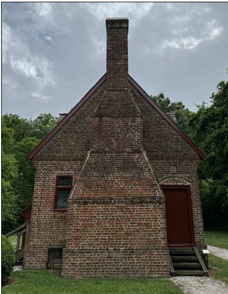
North side elevation, May 2024. Original window opening on the first story and original cellar window opening to the left of the chimney. Original doorway to the right of the chimney. Note glazed headers following the rake of the roof.
