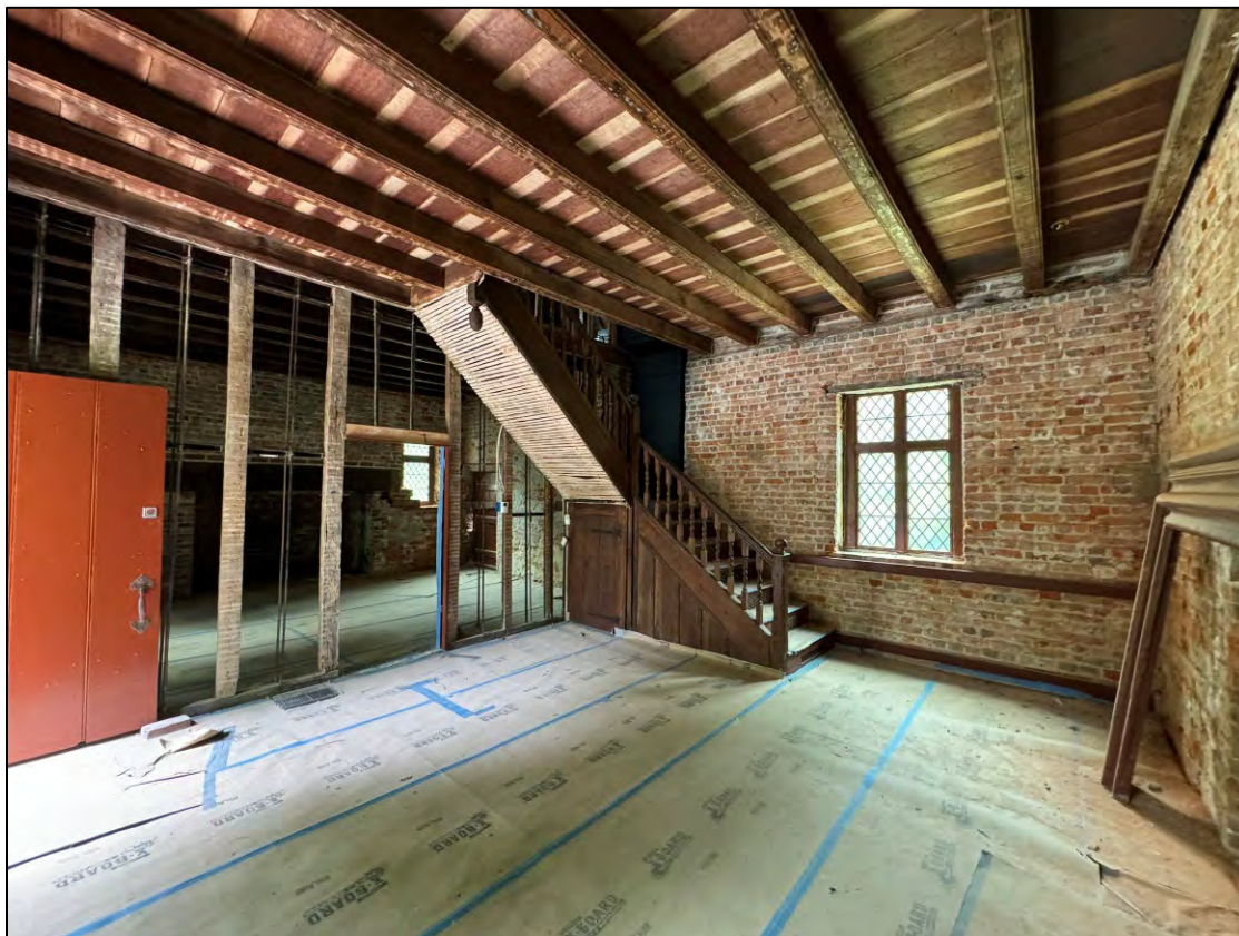
Hall. Front entrance is the open door leaf seen on the left. May 2024.
