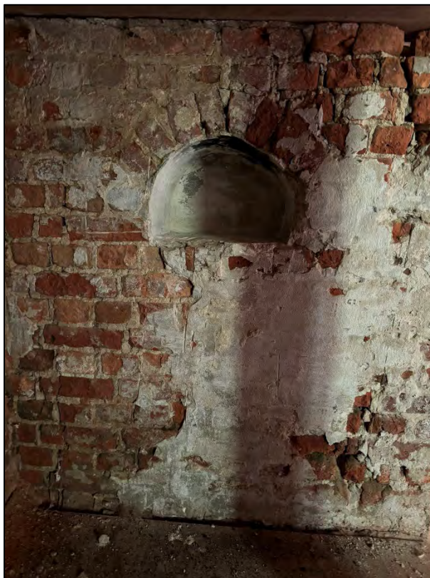
Parlor/dining room fireplace, warming niche on the east wall of the firebox. May 2024.
