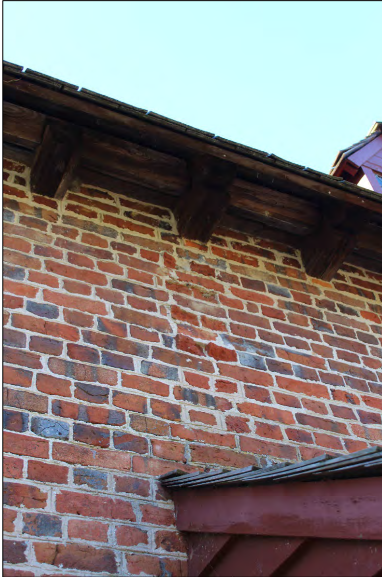
Evidence of missing rear wing. Note broken bricks in the middle of the photo. December 2023.
