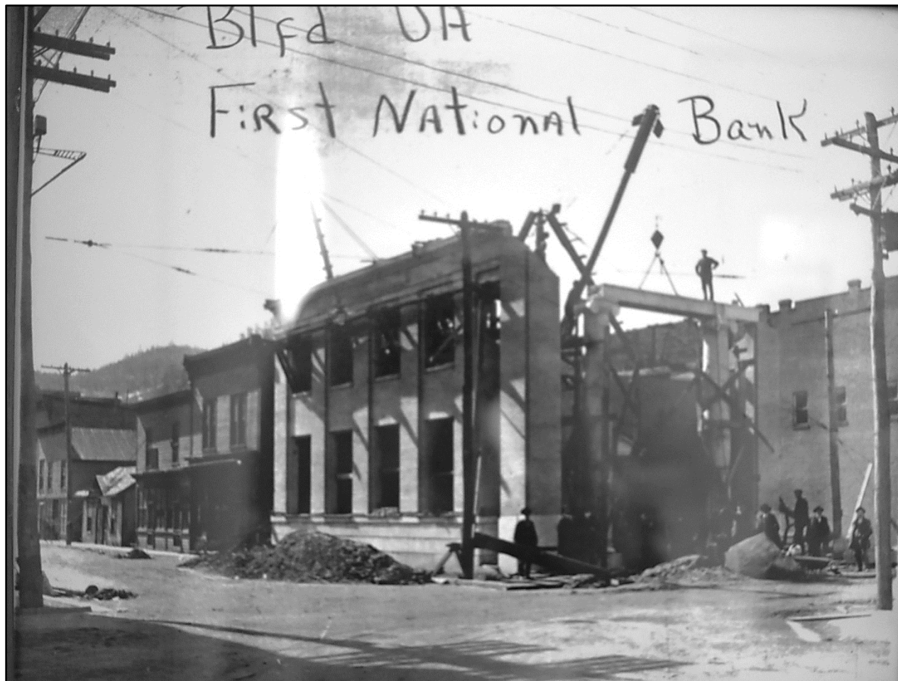
Figure 8. First National Bank at Graham Under Construction, ca. 1916. Source: Graham Historical Society, Sanders house, Bluefield, VA
