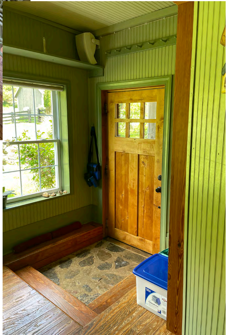
PHOTO 26 DATE: May 2024 DESCRIPTION: First Floor exit in kitchen in rear addition, view northwest.*
