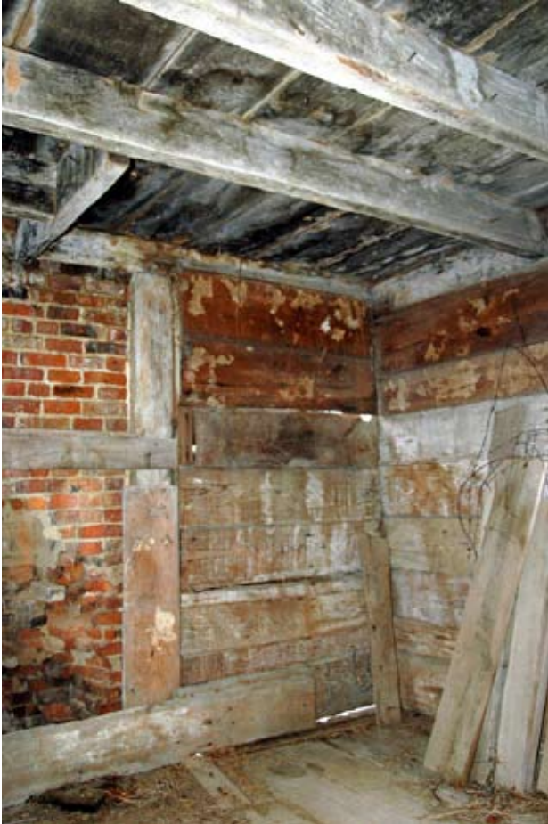
Figure 2. Closed stair opening.
