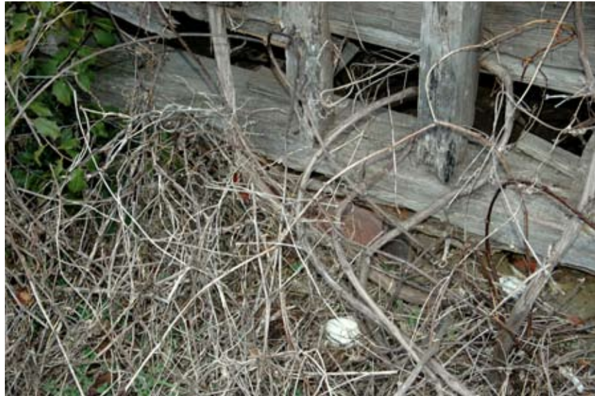
Figure 18. Failed framing: rear wall.
