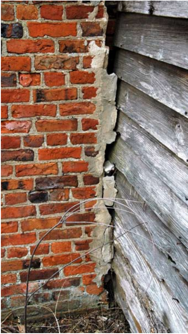
Figure 15. Chimney separated from building.
