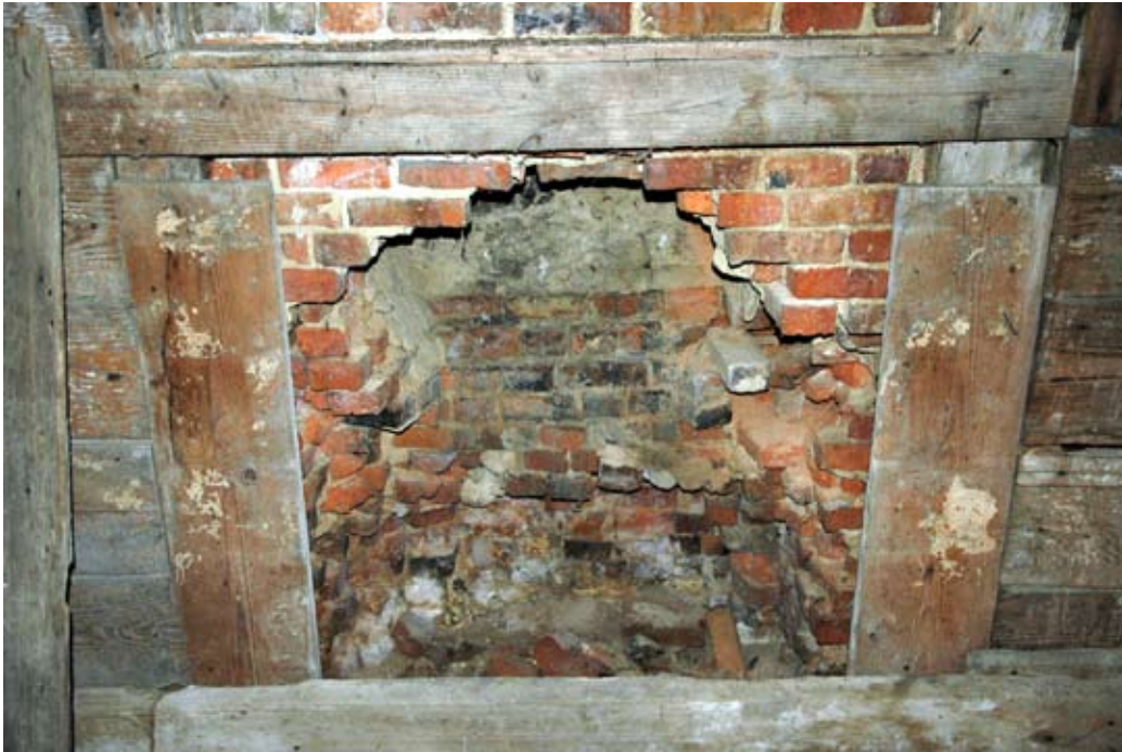
Figure 17. Collapsed fireplace jambs and arch.
