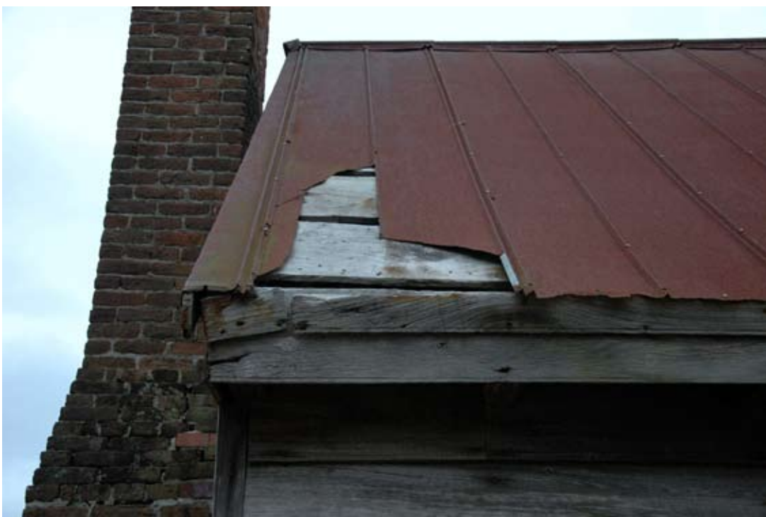
Figure 5. Failed roof covering.
