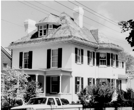
Owners of this Winchester home are replacing the slate roof a few pieces at a time over a number of years.
